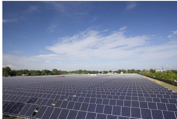
Exelon City Solar, Chicago, Illinois 10 MW SunPower T0 Tracker
