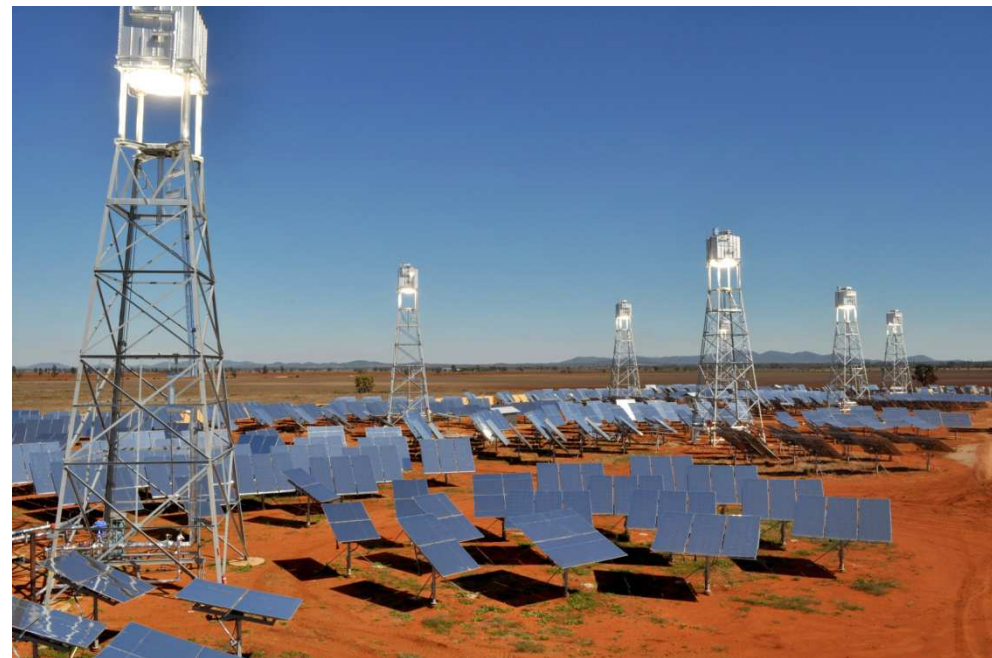
Graphite Energy's Facility at Lake Cargelligo, NSW
